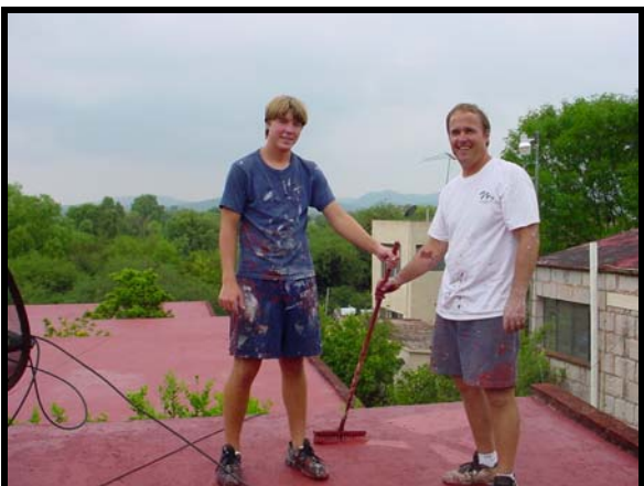
Mark & Koby Runge (father & son) show off their work of resealing the roofs of the homes of the elderly.
